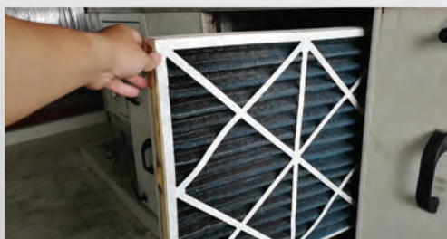
A/C Filter Replacement
