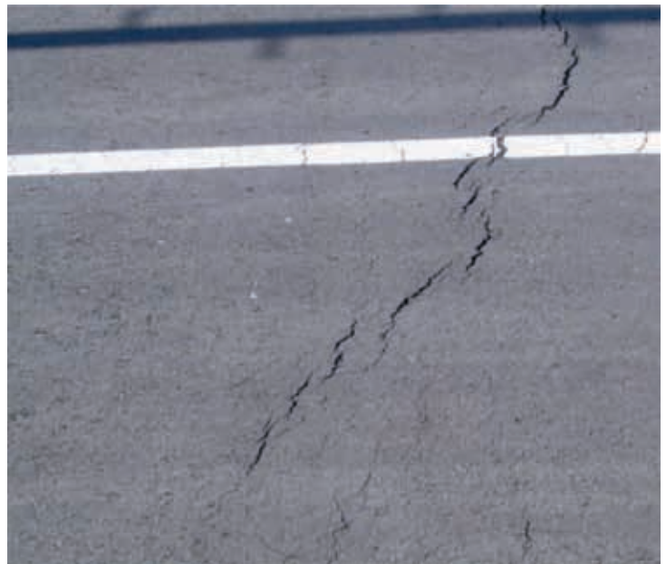
How to stop the spreading cracks in the Desert Vista parking lot will be under review.
