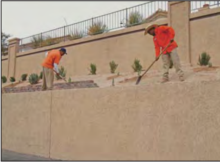
Landscape department crew members Marciano Oliva, left, and Oracio Ordonez reslope the area above the Desert Vista parking lot. New plantings will help to maintain homeowners' views, plus ensure a safe work area for staff.
