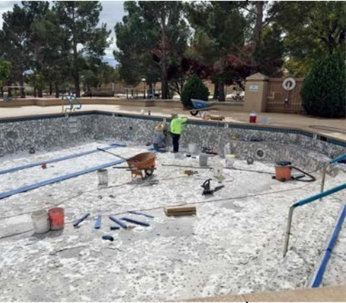
Workers apply new plaster to the outdoor pool at Desert Vista. The renovation project included several upgrades to tile and decking at both Desert Vista and Mountain Shadows' outdoor pools.
